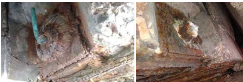
Figure 10 Corrosion on prestressing reinforcement anchors
