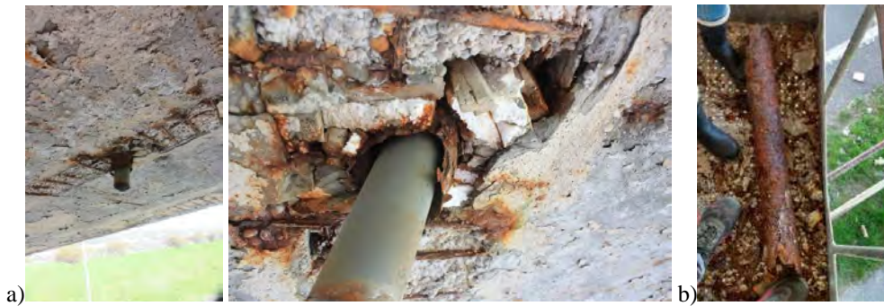
Figure 6 Detail of drainage pipes (a); original steel pipe after falling from polystyrene filled gap in lower flange (b)
