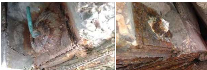
Figure 10 Corrosion on prestressing reinforcement anchors
