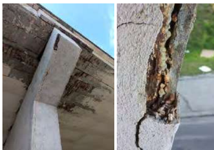
Figure 11 Corrosion of reinforcement and delamination of cover layer on pillars
