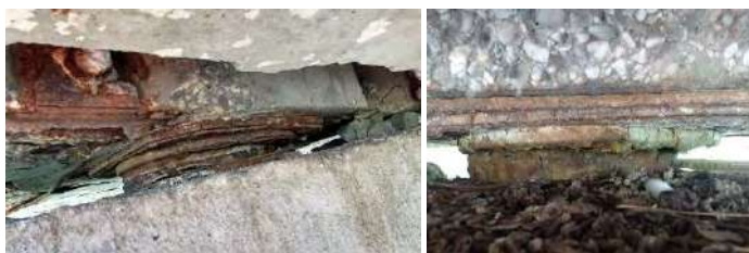
Figure 12 Corrosion of bearing and its deflection by the displacement of the superstructure
