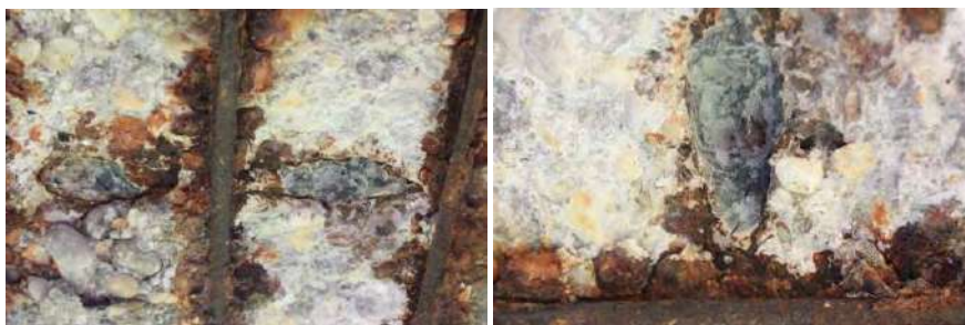
Figure 4 Exposed grouted corrodng duct - prestressing reinforcement was free of corrosion at the time of the survey
