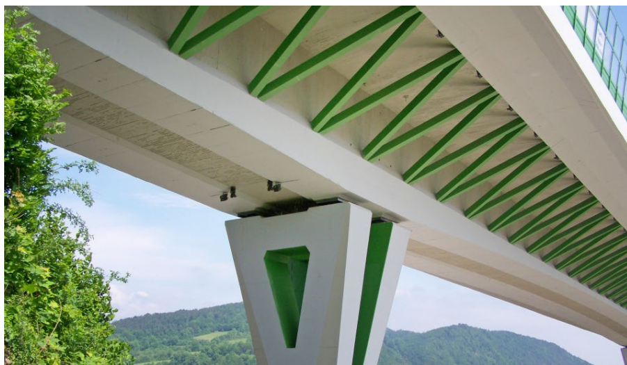
Underside of the the Považská Bystrica Bridge, an example of Slovak structural engineering
